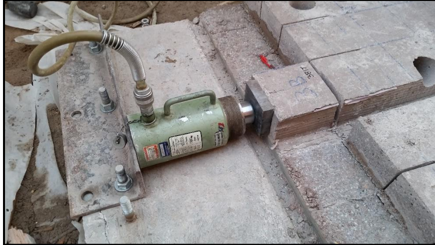
Figure 3-22 – Simplex RC306C hydraulic testing specimen on Slab 2A. On right, 1 in (25 mm) steel plate; on left, brace angle bolted to substrate
