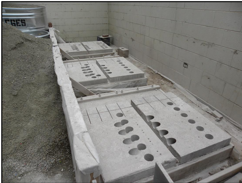
Figure 3-9 – As constructed view showing pull-off, direct shear, slant shear, and jacking test sampling locations. Background to foreground: Slab 1, 2, and 3
