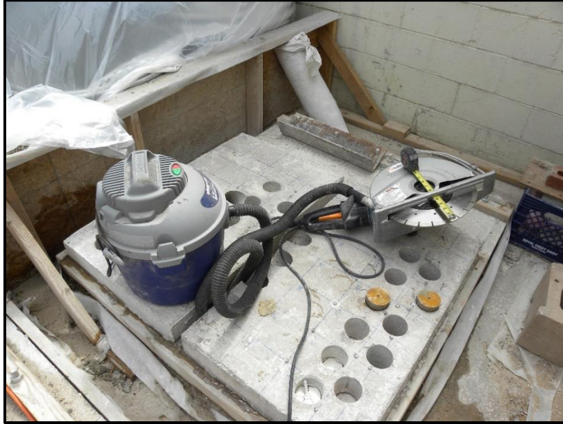
Figure 3-21 – Concrete saw and dust collection system
